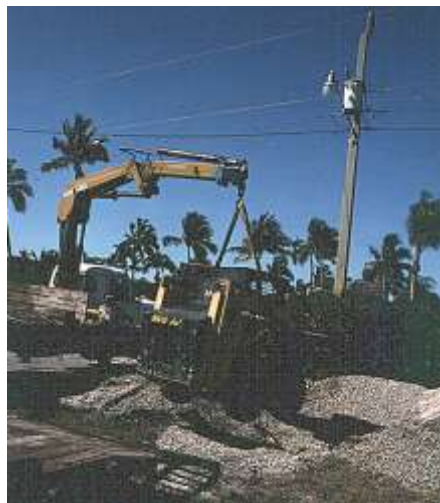
Construction Work on a Site: Typical examples of what you can see going on at a construction site if you are monitoring. Tree moving and other activities at the Olde Marco Inn.
